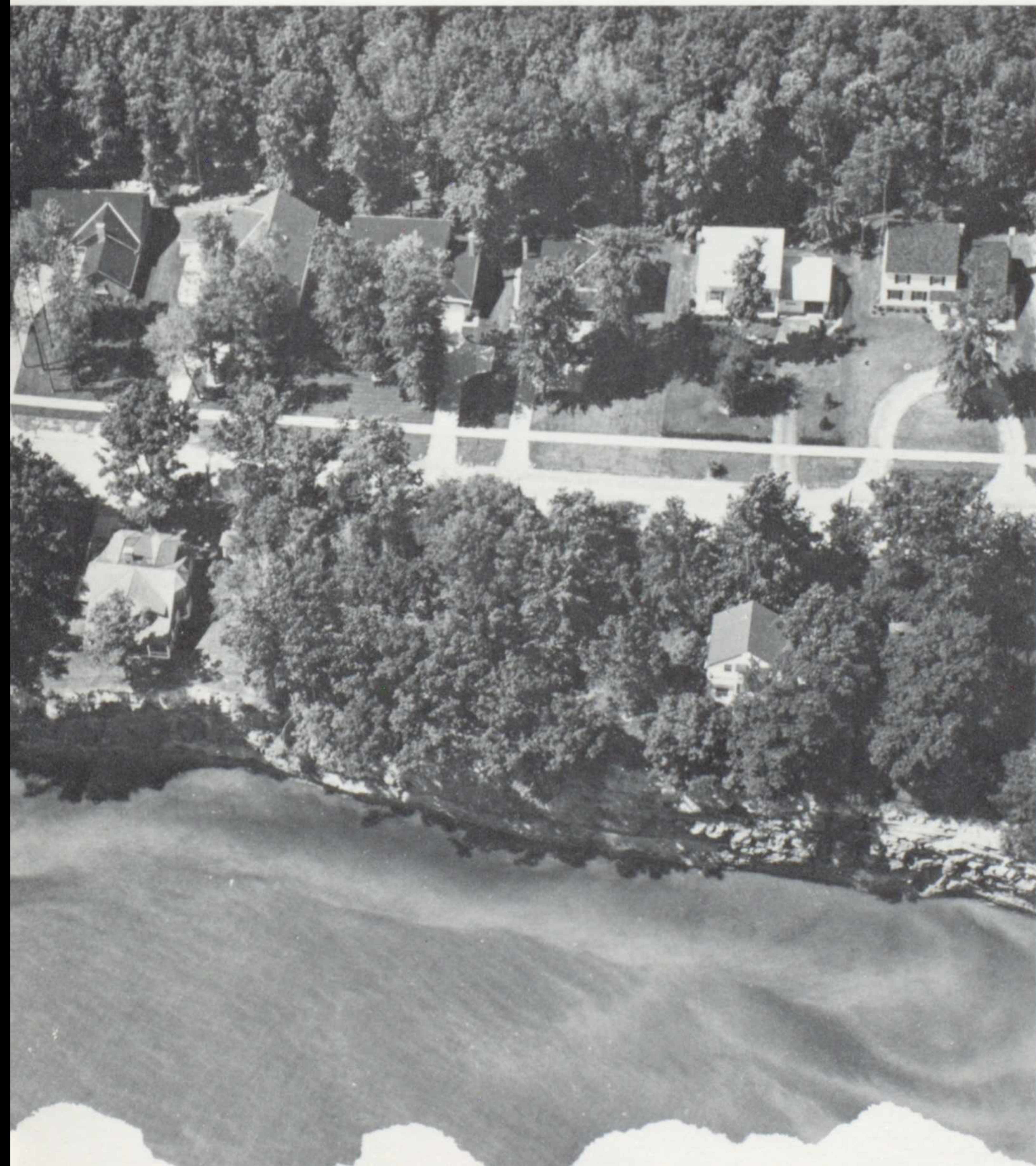
High water and unrelenting currents visibly tear away at the defenseless shoreline to the chagrin of homeowners.
