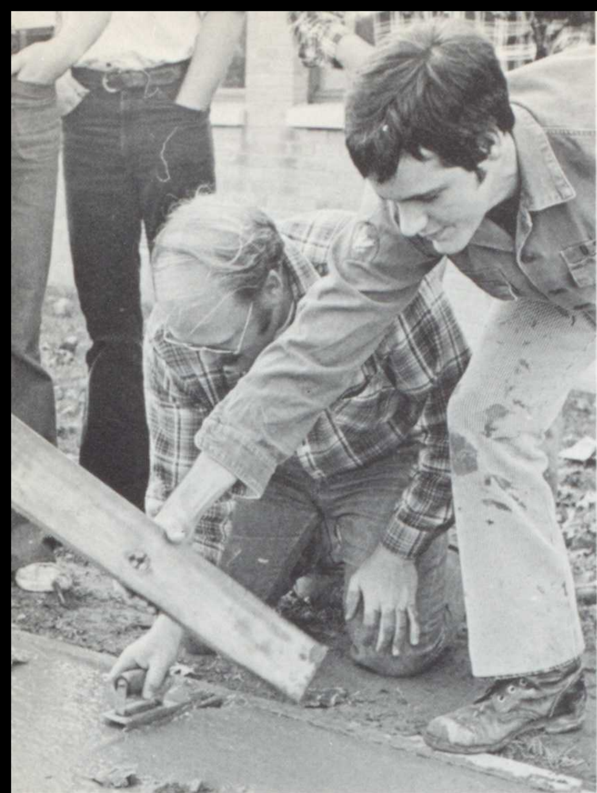
Among fallen leaves, shop teacher Alan Schneider and Rich Krueger smooth concrete near the newly added shop wing.
